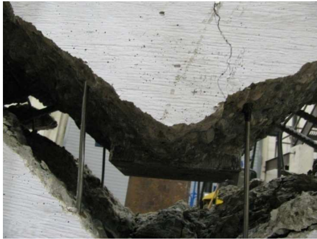
Figure 3- 8 Breakout cracking initiation from the plate ends
