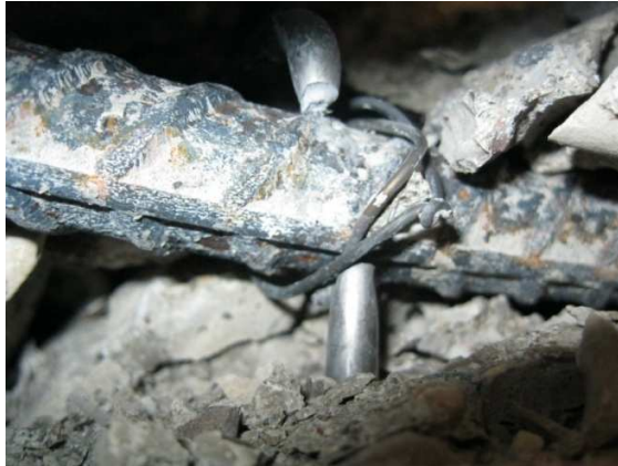
Figure 3- 10 Stirrups failure by necking after the breakout cone formation
