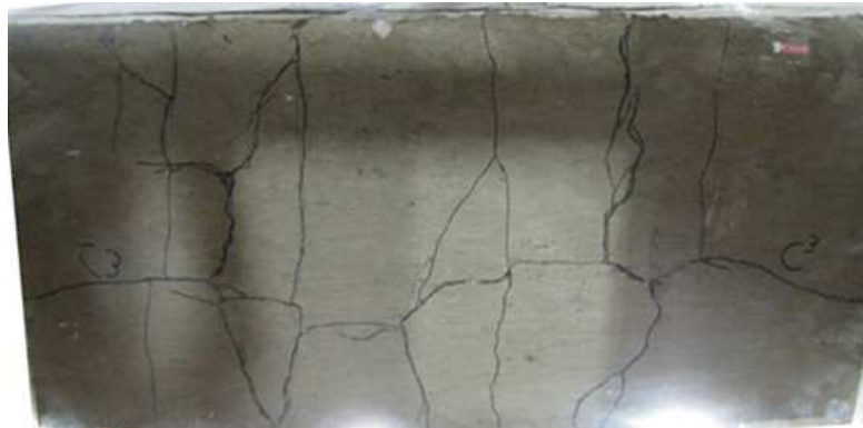
Figure 6- 8 Observed splitting cracks in beam C3
