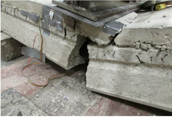
(a) FMA2-1 (strand rupture).
