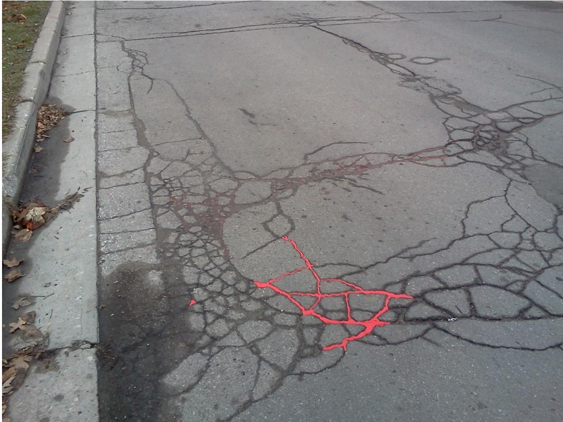
Road Work, William St. documentation of site II. Plasticine in asphalt. Dimensions variable, 2012-13.
