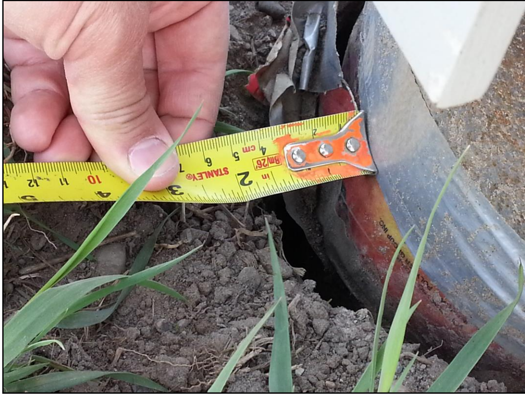
Figure 5 - 13: An image of the developed gap behind pile PA1 at the end of the cyclic lateral testing
