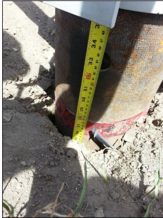
Figure 7 - 15: A field image of the developed gap behind pile PA1 at the end of the cyclic lateral testing
