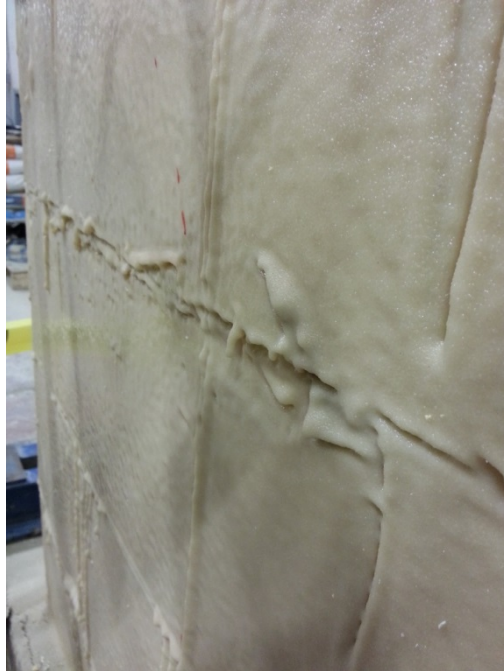
Figure 5.13: Polyurea dripping on the wall surface
