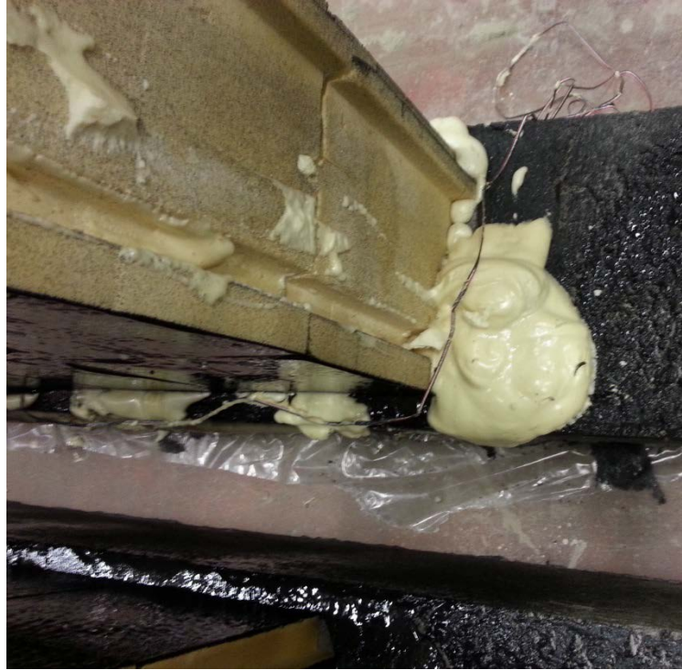
Figure 5.10: leakage of the liquid foam
