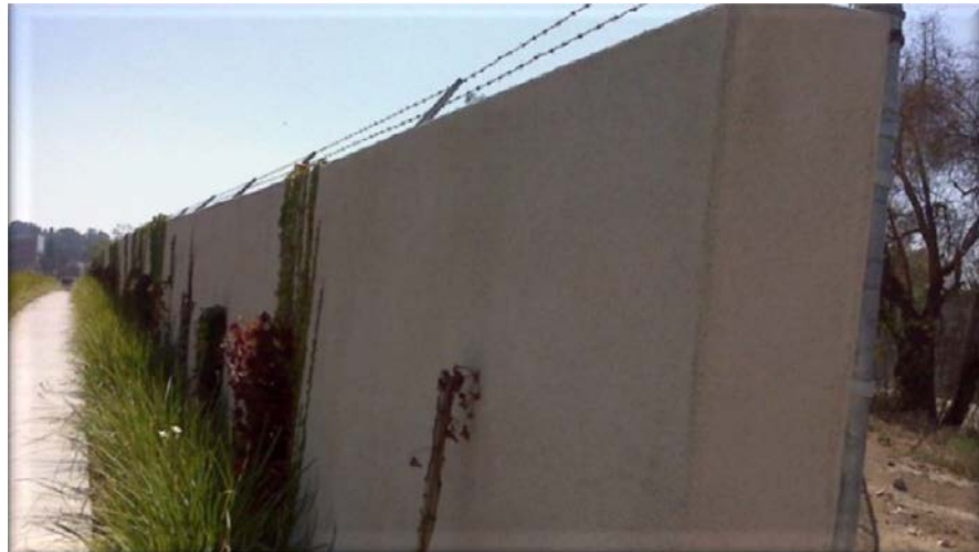
Figure 5.14: Utilization of Poly-block with concrete cores in construction project of West Los Angeles Community College (Lexicon website)
