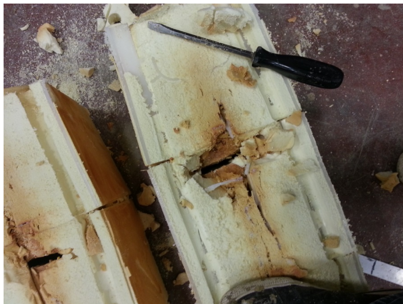
Figure 5.9: Crack in wall cores due to leakage
