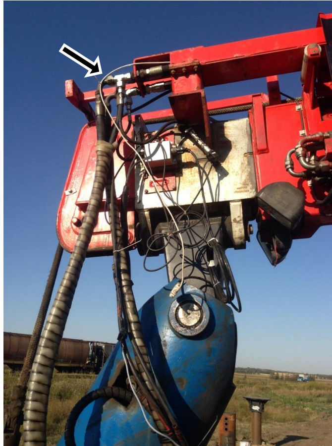
Figure 4-5: Hydraulic Pressure Transducer
