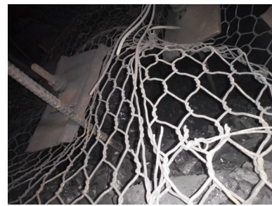
(c) 锚杆、锚索失效
