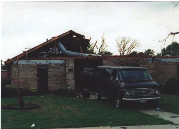
Figure 1.1 - A reference for degree of damage six (from Texas Tech University, 2006).
