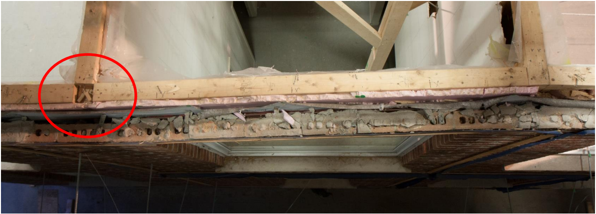
Figure 5.3 - Wall D10-F10 as the joint as D10 is failing.
