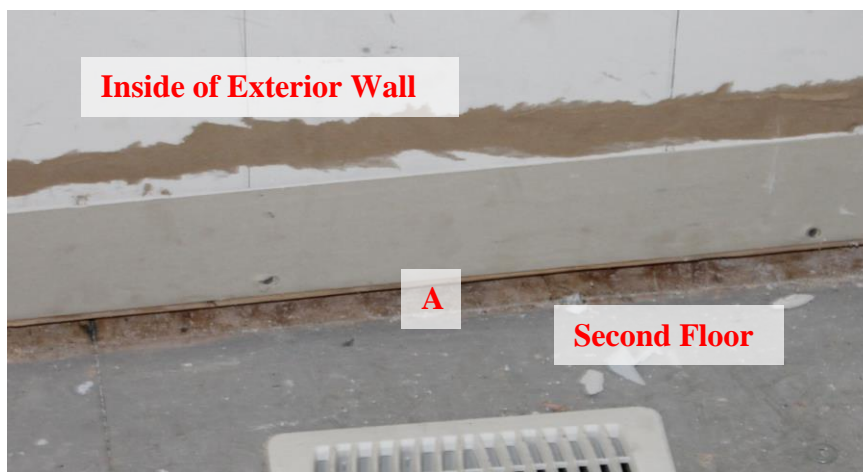
Figure 8.2 - Second storey floor-wall connection post failure
