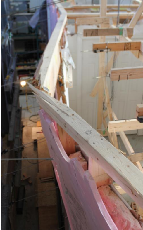
Figure 6.9 - Wall section B1 immediately after failure.
