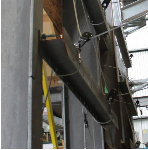
Figure 3.8 - A separation beam installed on the reaction frame. The pulleys redirect the cables from the house towards where they join.
