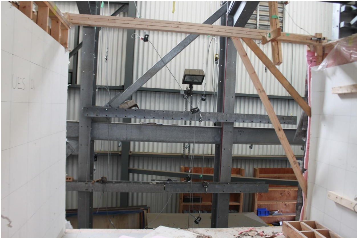
Figure J1 - The false top plate installed at A10-E10 to increase the stiffness of wall A1-J1.
