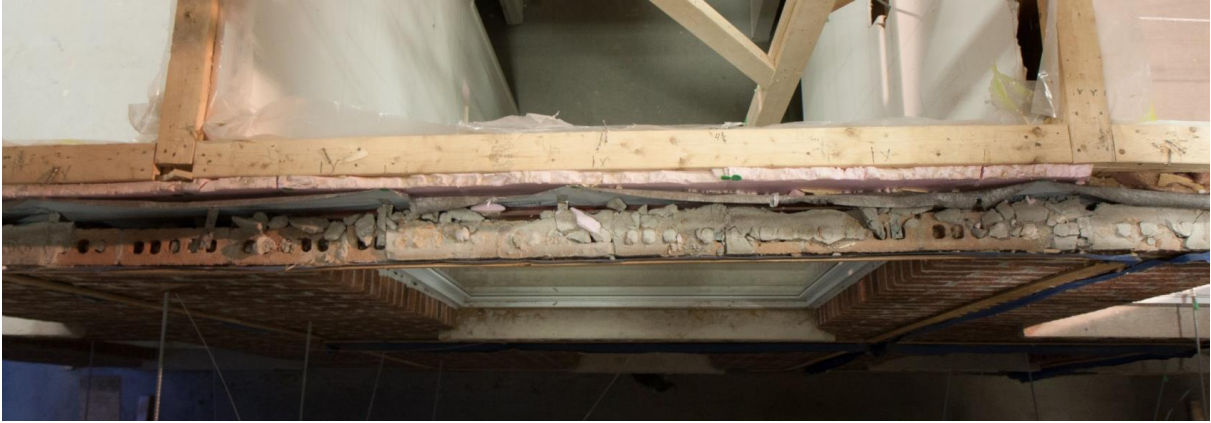
Figure 5.2 - Wall D10 - F10 loaded immediately prior to failure.
