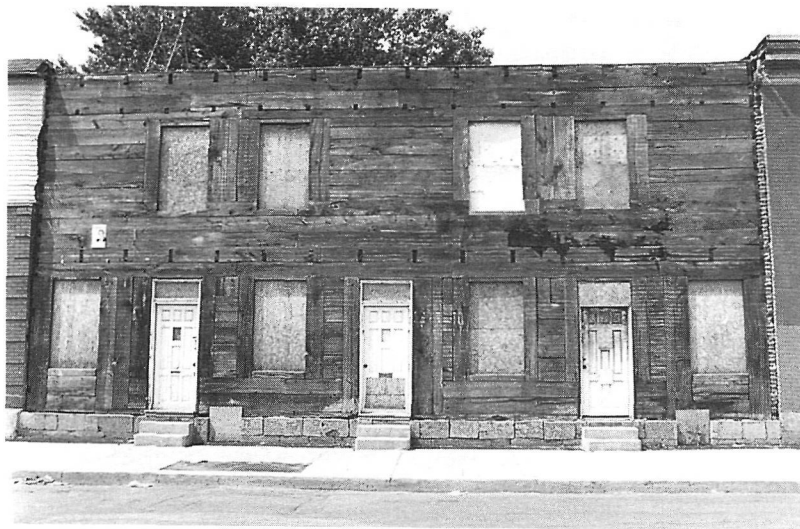
Working-class homes of the 1872 boom were still of plank construction “pièce sur pièce” as shown for a double-duplex on Liverpool street; the brick cladding has been removed, for replacement.
