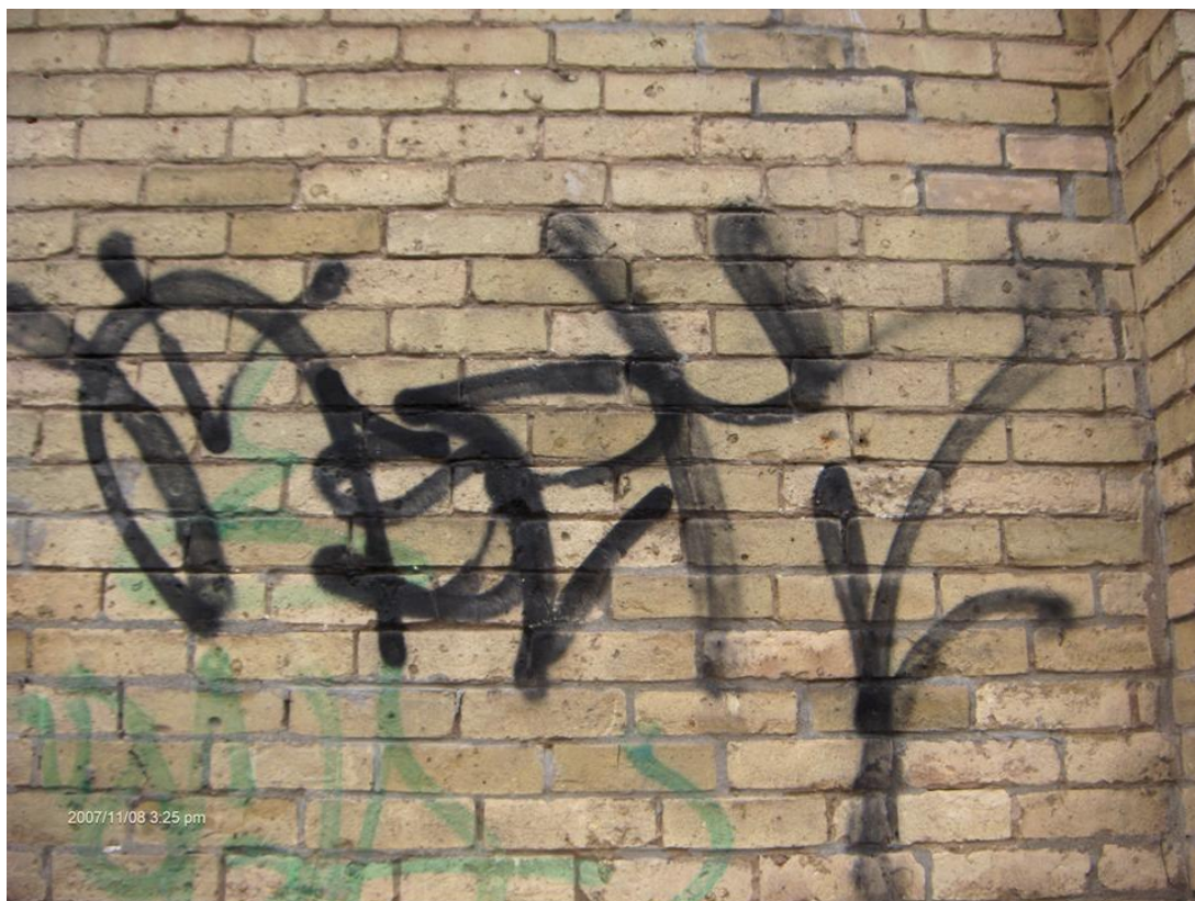
Figure 4.1: Graffiti on local building
