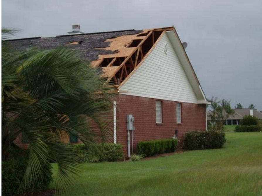
Figure 1.1: Failure of roof sheathing above gable end, source: www.floridadisaster.org
