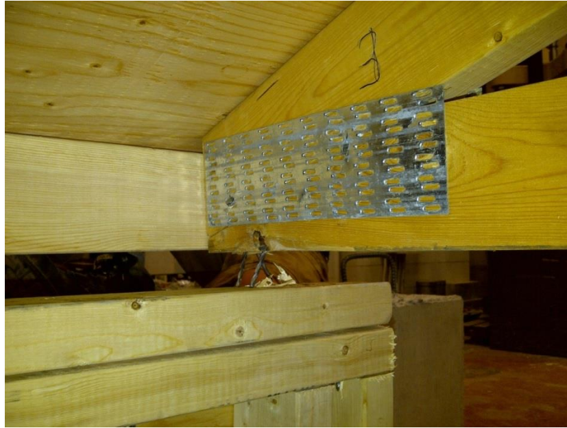
Figure 5.11: Failure of connection W1-L3 after sudden withdrawal during control experiment
