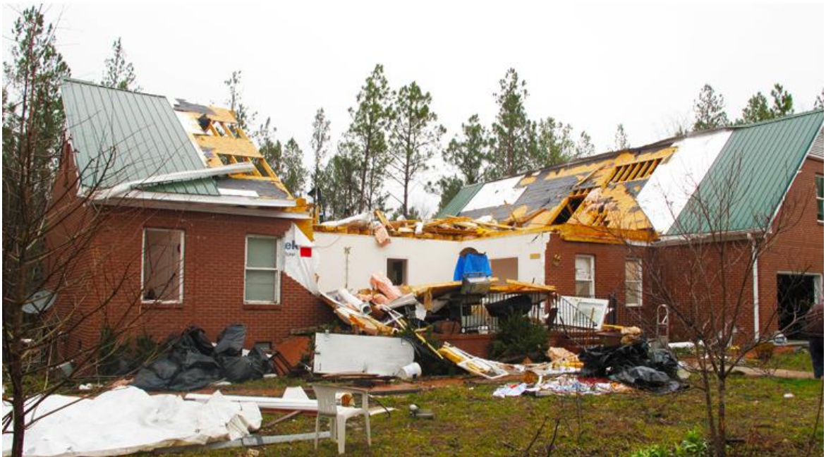
Figure 1.2: Example of roof system failure after multiple RTW connection failures, source: www.Disastersafety.org
