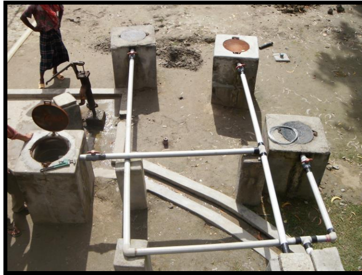
Figure A2: Assasuni field site well layout (square concrete, raised structures are injection wells, metal hand pump in upper-left corner is the extraction well).
