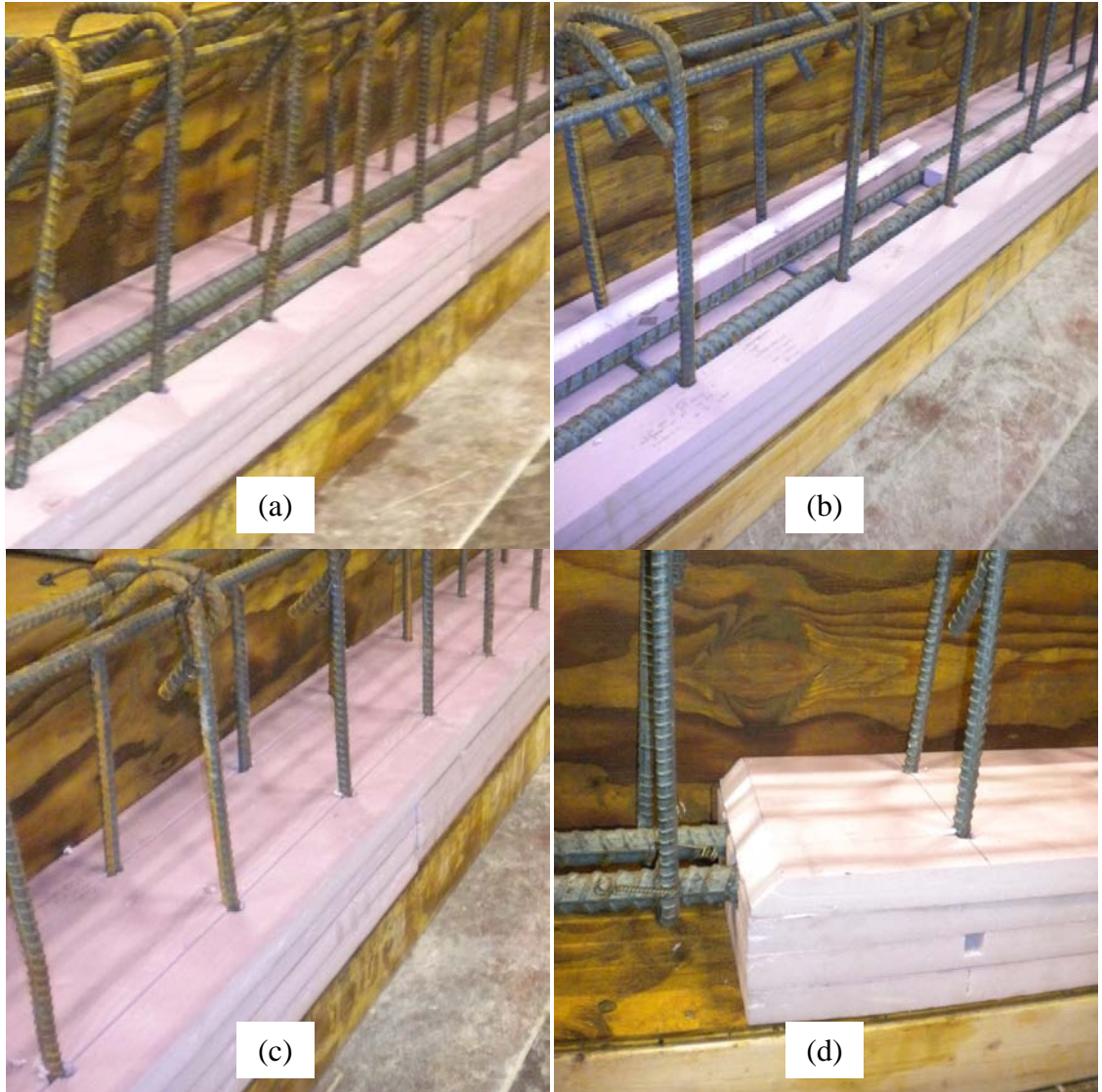
Figure C-9: Foam Insulation Void Placement: (a) Stirrups and Flexural Reinforcement Placement, (b) Layer 3 Placement, (c) Layer 4 Placement, (d) Beveled Edge of Layer 4.
