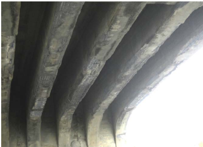
Figure 1-1: Typical Deteriorated Reinforced Concrete Bridge Girders.
