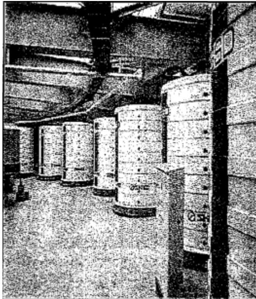
Fig. 1.15. Stacks of Cylindrical-TLD MMDs Installed in SYPH (from Tamura et al. 1995)
