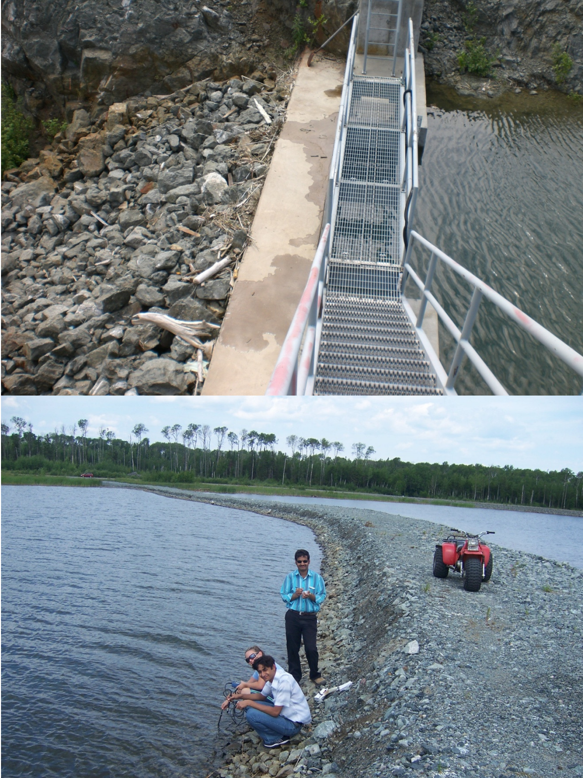
Figure IV-3 Pictures of open spillway (outlet) and a wave break, which separates the cells in tailings pond
