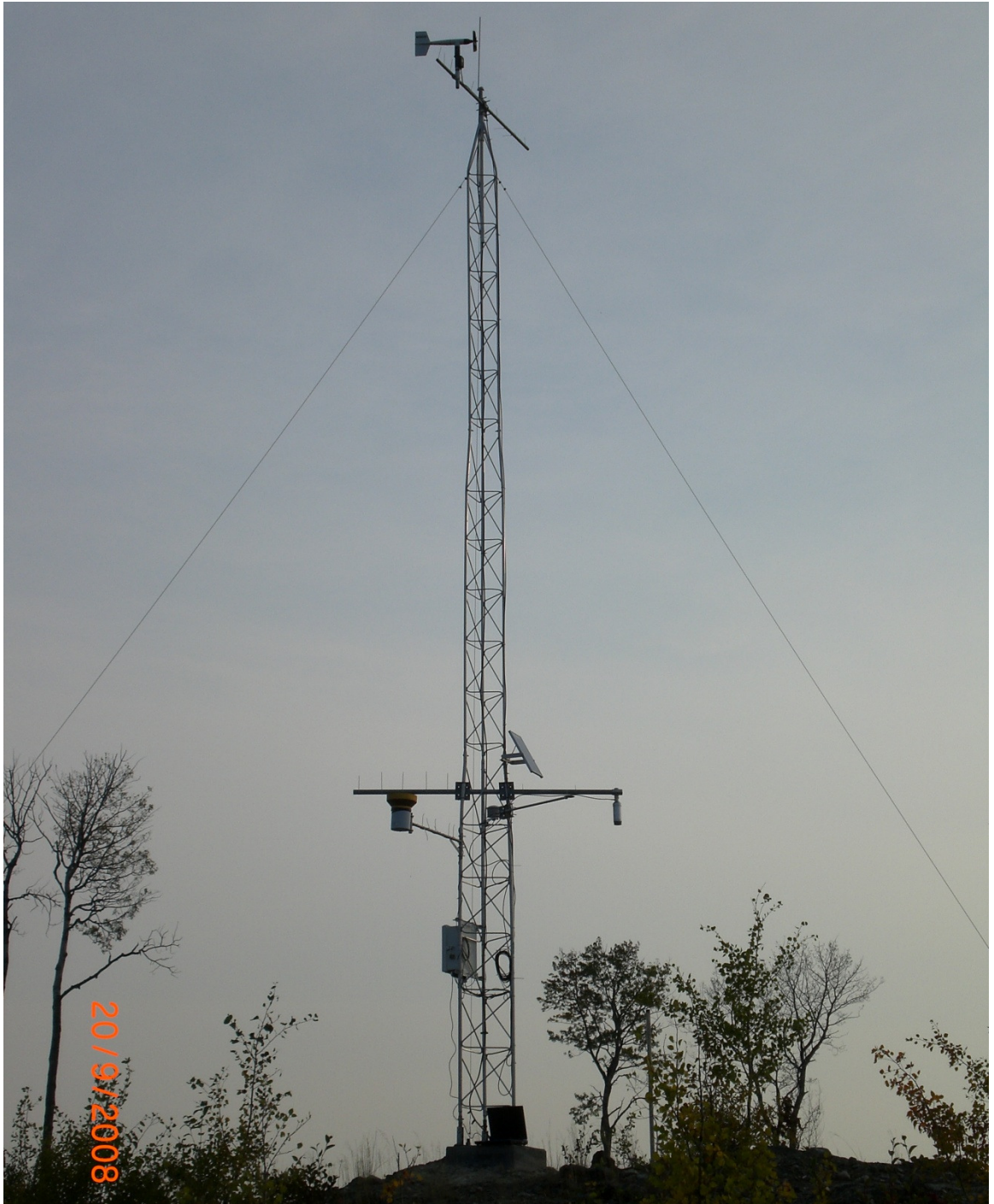
Figure IV-4 Weather station installed at the Shebandowan tailings storage facility
