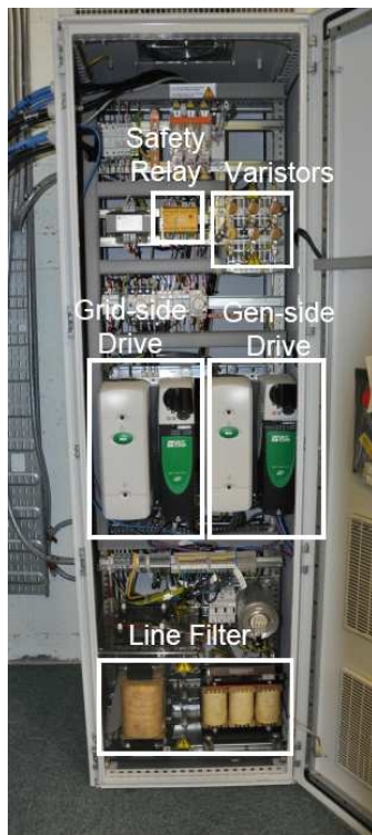
Figure 8 Regenerative Drive Panel
