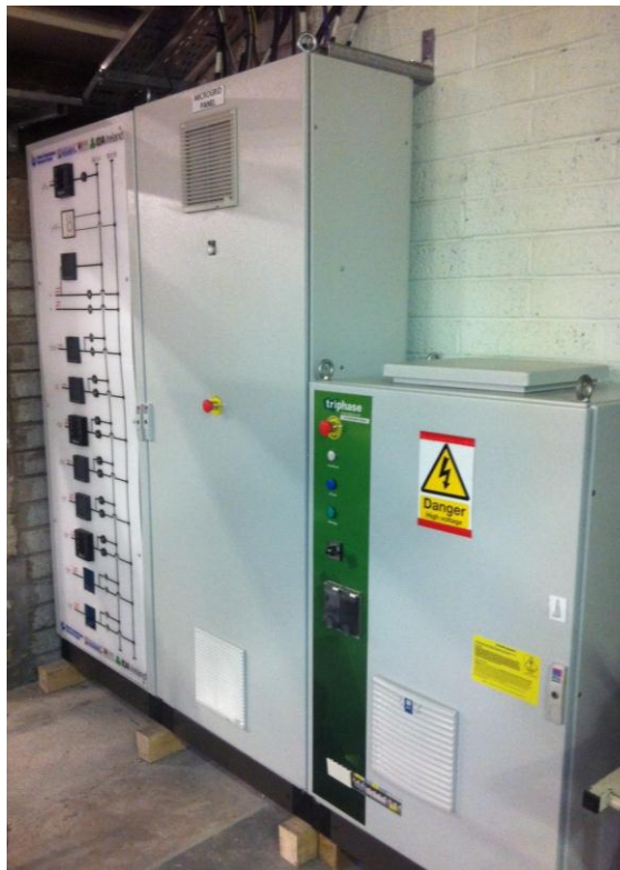
Figure 5.12: Microgrid panel and Triphase panel installations
