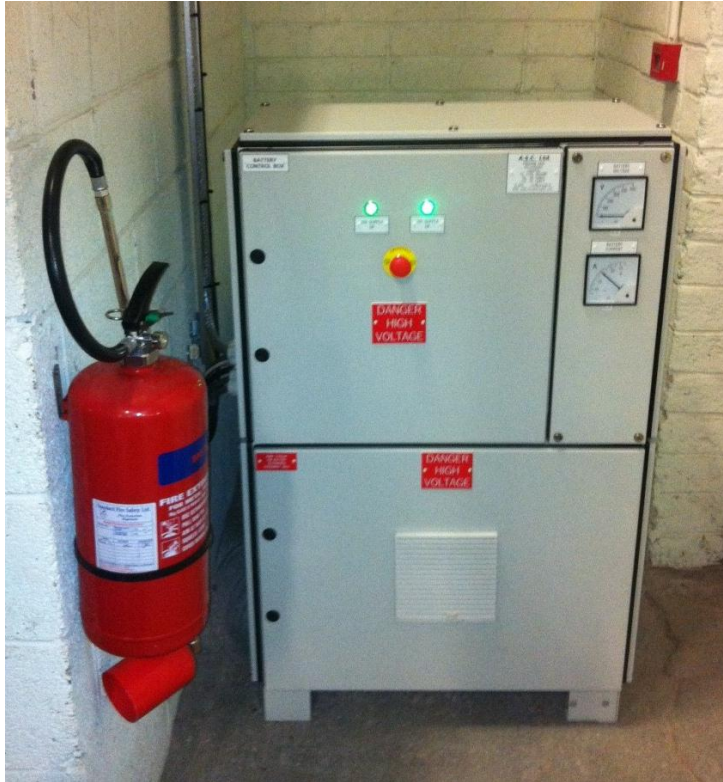
Figure 5.9: Front view of the high voltage battery enclosure including panel with associated control electronics
