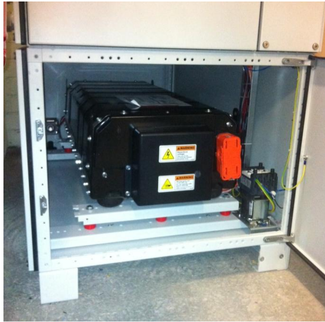
Figure 5.11: Battery enclosure internal view
