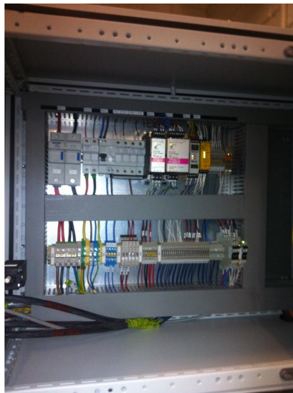
Figure 5.10: Battery panel internal view
