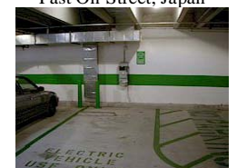
US Disabilities Compliance EV Parking Bay in a MSCP
