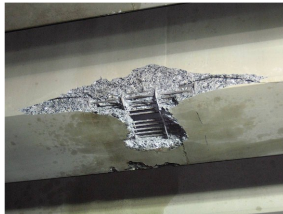
Figure 2 – Photograph of Impact Damage
