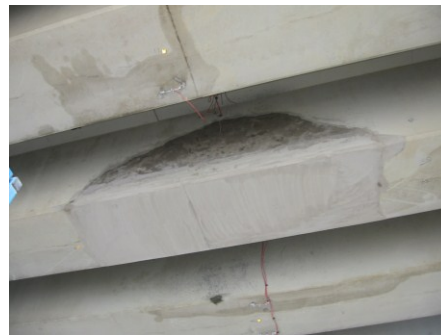
Figure 6 – Repaired Section of Damaged Beam
