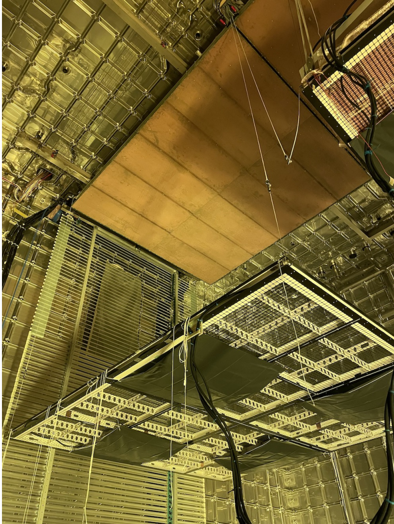
Figure 8.1. The inner volume of NP02 during installation of the FD2-VD Module 0 detector. The two top CRPs are visible, along with one cathode equipped with four X-ARAPUCAs , the downstream cathode is temporarily elevated and two X-ARAPUCAs on the upstream wall are visible behind the upstream field cage (the downstream membrane wall X-ARAPUCAs are not visible). All of the X-ARAPUCAs are covered by temporary bags.
