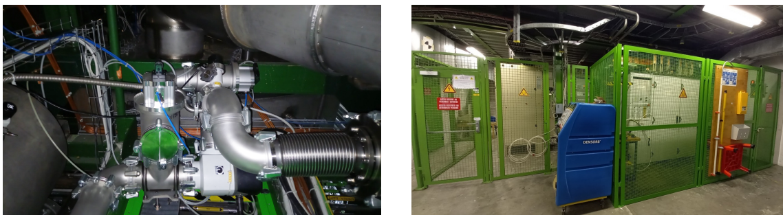
Figure 3. Photographs of a part of the new vacuum pumping circuit (left) and of the new CMS FWT system installed in the CMS service cavern (right).
