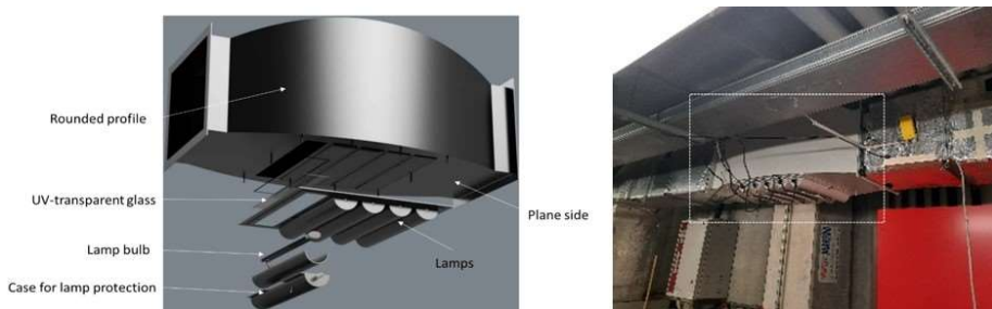
Fig. 1. Left: exploded 3D image of the system designed for installation in the existing ATU duct at CSMT Headquarters and adapted from (Lombini et al., 2022). Right: Prototype installed at CSMT Headquarters.
