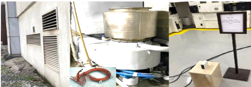
Figure 5. (a) Intake external air scenario. (b) Refrigerated hydrodynamic precipitator. (c) internal monitored environment. Source: authors in the field. Rio de Janeiro/BR, 2023).
