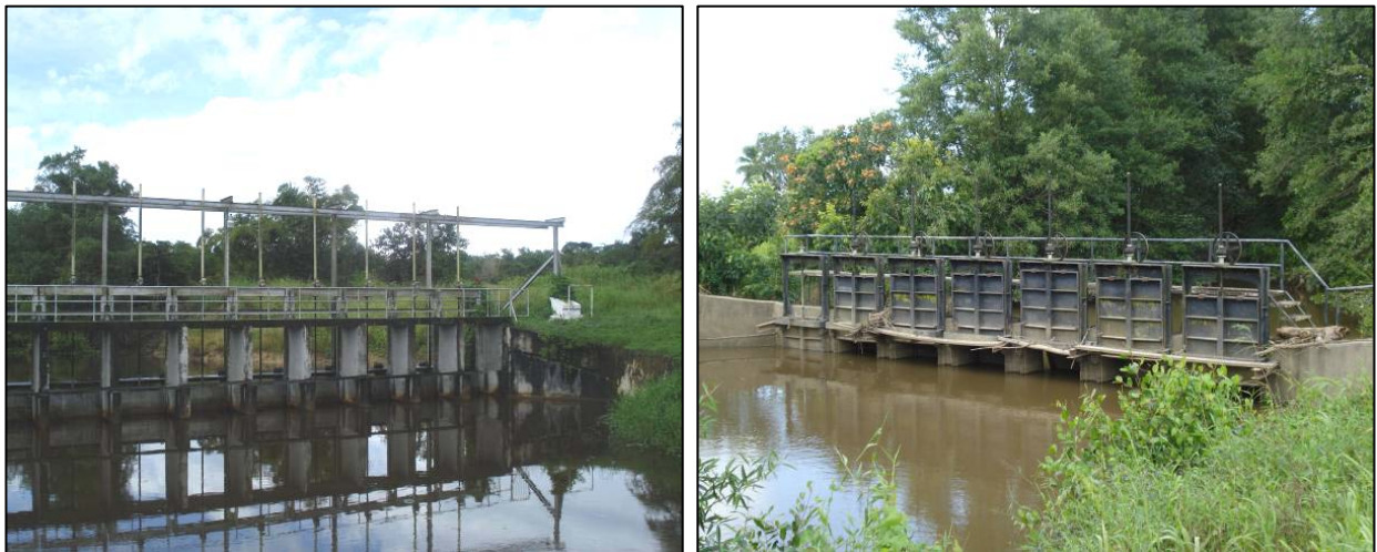
Figure 3: Water control gates installed in the lagoon to regulate the salt water intrusion and flooding.
