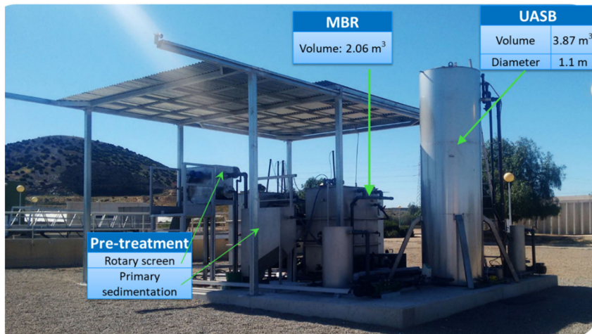
Figure 5.24 Image of the SIAM® prototype (using the second development) operated in the sewage treatment plant of the city of Cartagena (Spain), in the frame of the European Union Life Siamec project.
