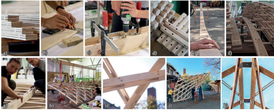
Fig. 7: Top Row: Prefabrication. 12 \times 100 mm planks (a) are marked (b), drilled (c), and coupled with 24 mm studs (d) into pre-bent (e) beams (f). This process embeds the geodesic curvature. Bottom Row: Assembly and Erection. The asymptotic beams and geodesic planks are interlaced into flat segments (g), and deformed into the doubly curved shape (h). The combination of asymptotic and geodesic planks (i) creates a stiff shell, that is transported (j) and assembled (k) on site.
