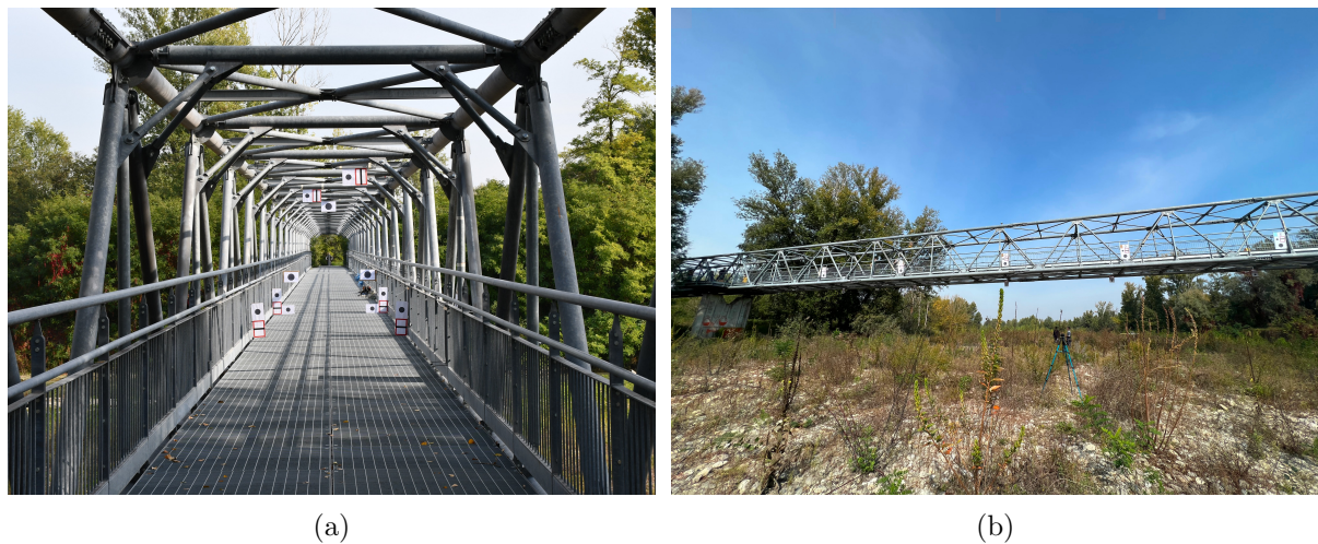
Figure 1: (a) View along bridge axis and (b) Side view of the structure and its targets.
