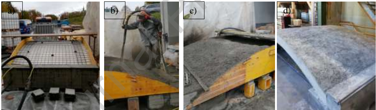
Fig. 11. V-SE: a) formwork, b) projection process, c) after projection, d) after curing.
