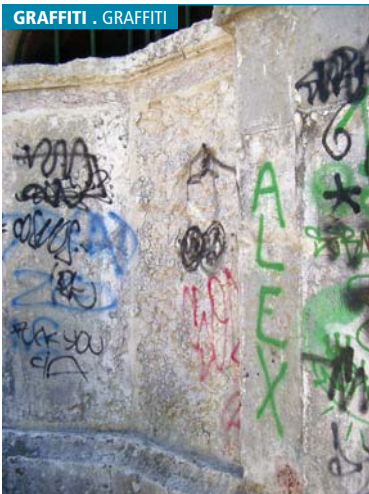
Graffiti in the west abutment of the Aqueduct built in limestone.
