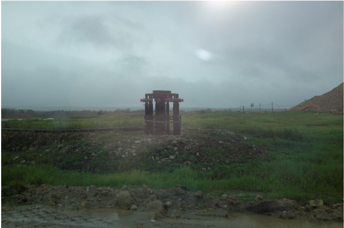
Photograph 78: Black plastic flare-pipes at the Lucas Heights Resource Recovery Park
