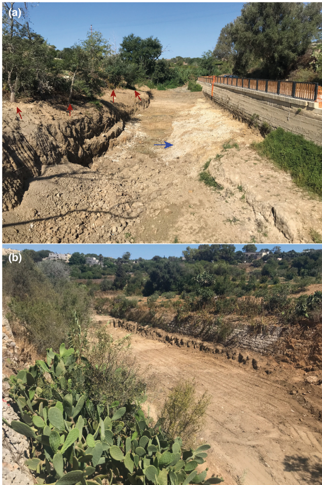
FIGURE 2 Pictures to demonstrate the constraints on efforts to ensure no refuges were left for crayfish during mechanical excavation. (a) Red arrows mark a handful of protected White Poplar Populus alba trees, which meant the bank could not be excavated (note the blue arrow shows where bedrock was struck during excavation). (b) Shows the traditional rubble wall alongside the valley system. A 0.5m buffer was left along such walls to retain their structural integrity. Crayfish could have survived in burrows alongside these buffers.
