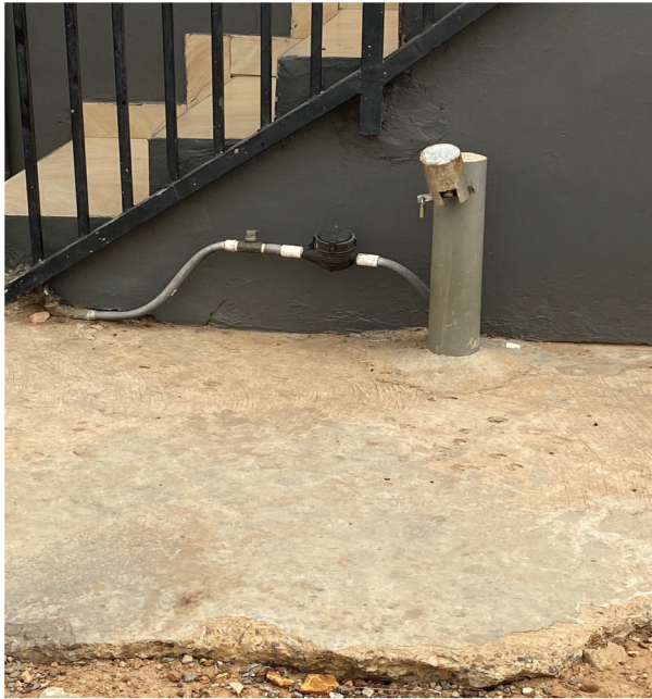
Figure 3. Private water connection in Dodowa supplied by GWCL (March 20, 2020).
