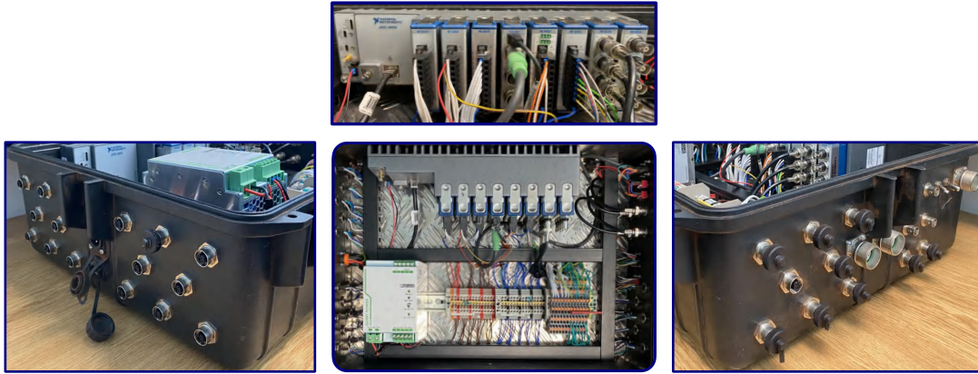
Figure 3.6: Data acquisition system with I/O modules and bulkhead connectors.
