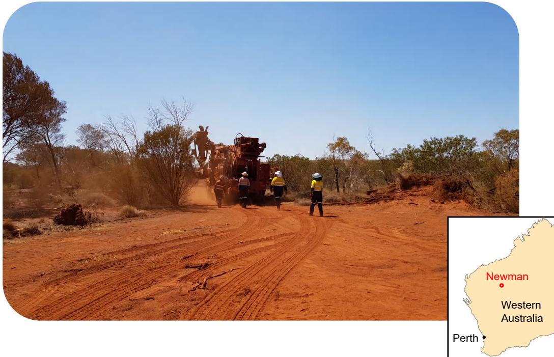
Figure 3.1: Drilling rig being mobilised to the desired location. Rio Tinto mining site area located near Newman (approximately 1177 kilometres from Perth (capital of Western Australia)).
