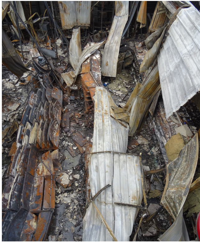
FIGURE 1 Overhead photo taken through a gap in the collapsed roof taken from a hydraulic platform.
