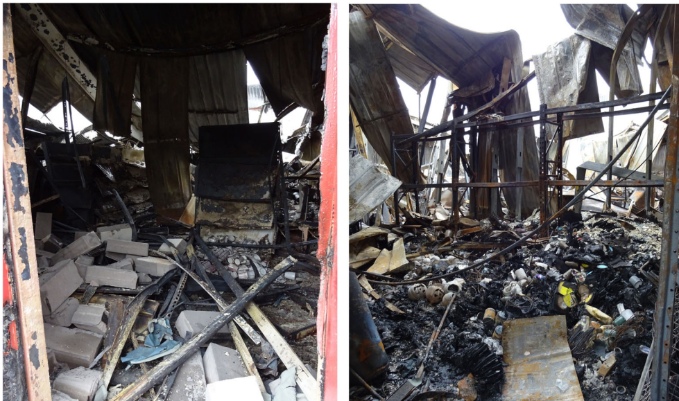
FIGURE 2 Extent of structural collapse and burnt debris in a commercial retail unit fire.
