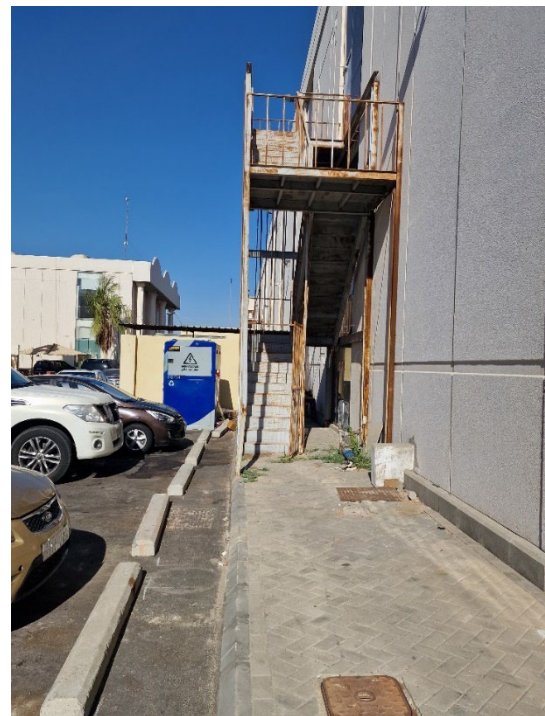
Figure 6-31. A typical example of an external staircase that obstructs sidewalk continuity.
