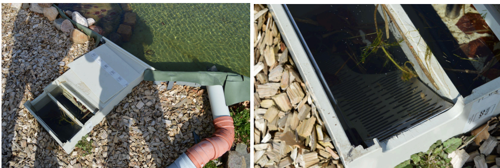
Figure 9. Skimmer pump system removing the floating debris from the pool. (The picture was taken by: Ernő Tóth-Pál)
