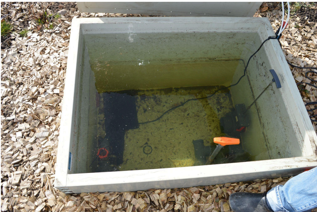
Figure 10. Submersible pump chamber (The picture was taken by: Ernő Tóth-Pál)
