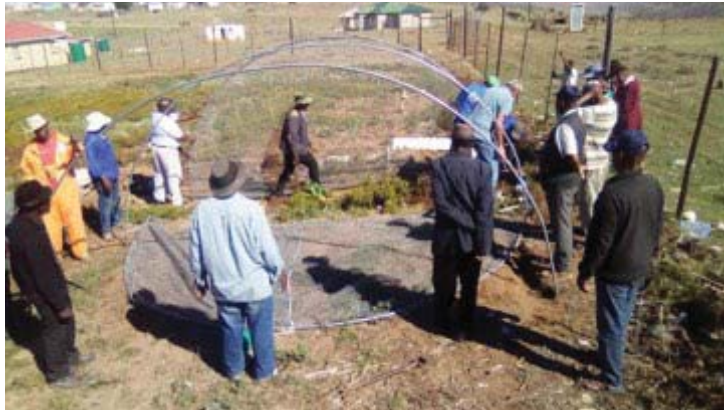
Figure 5.4. IBLN Members work with the CSA team to erect a shade-cloth tunnel at Xhukwane, Eastern Cape
