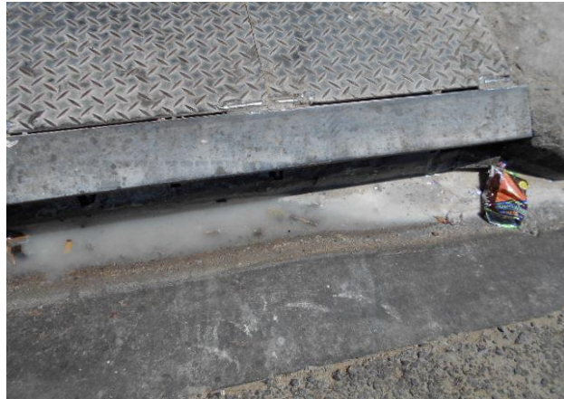
Figure 7: Covered drain to avoid pollution
