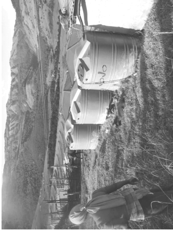
Tanks storing rain water collected when it flows over the ground. Note: to get the top of the tanks lower than the catch pit it was necessary to partially bury the tanks
