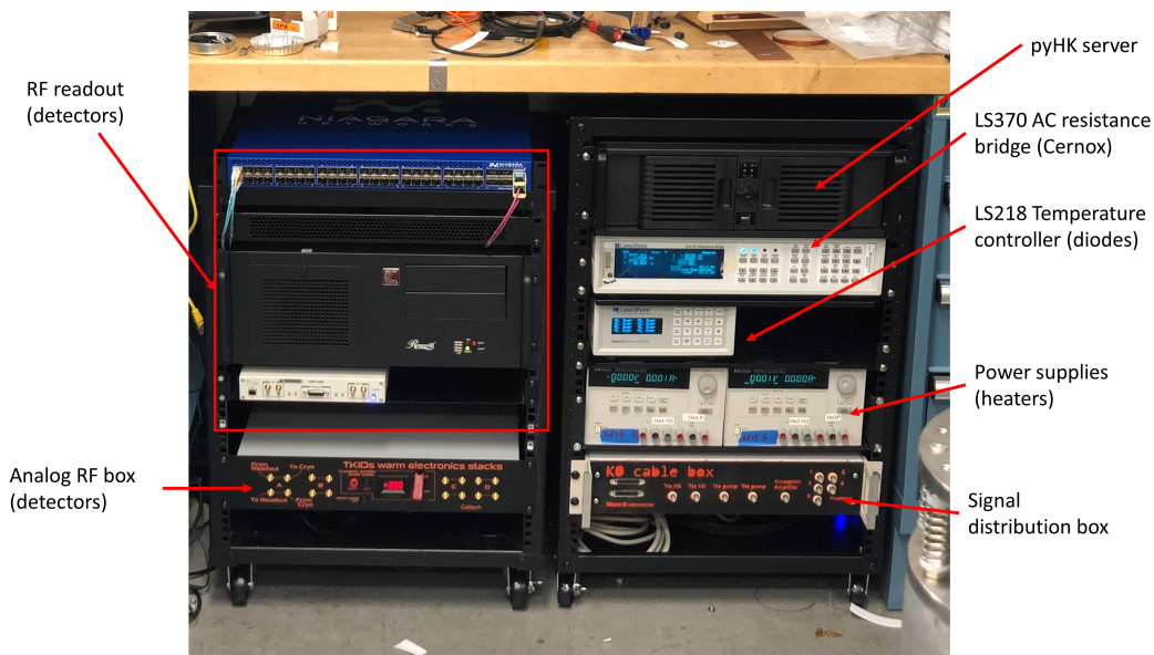
Figure 3.10: Instrument cluster for K0/sK0 housekeeping and detector readout. On the left rack there is the room temperature RF readout chain that includes an Ettus SDR, a GPU server, a packet broker and a box containing RF amplifiers, filters and linear power supplies. On the right rack there is the housekeeping server, the LS370 for controlling the Cernoxes, the LS218 for reading out the diodes, the switching power supplies for operating the heaters and the signal distribution box. This picture was taken during the commissioning phase of the lab.
