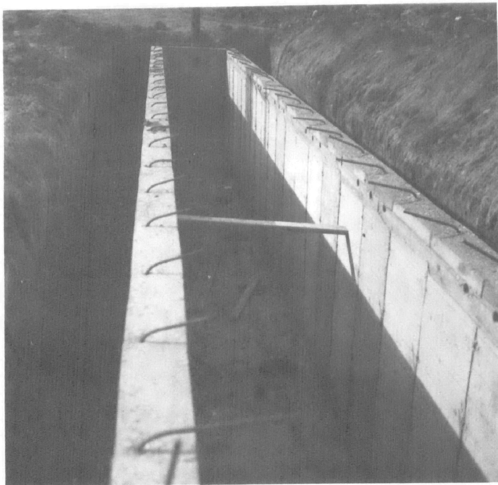
Figure 5. Access tunnel, experimental feedlot, prior to backfill and completion of feeding apron.
