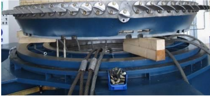
a) Upper row of ventilation ring vanes
