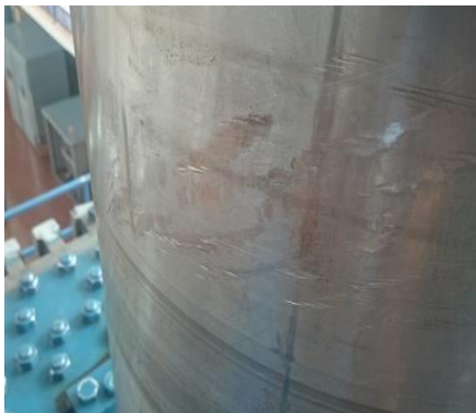
a) Appearance of mechanical damages in area 1
