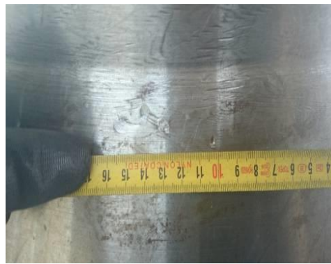
b) Appearance of mechanical damages in area 2
