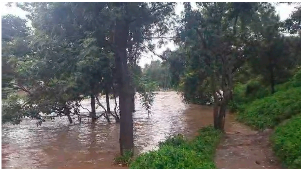
Figure 12. Screenshot from a local resident's video shared on a community WhatsApp group, accessed on 7 th May 2024. This should show Fatima Bridge, a Kandisi River crossing for cars and pedestrians. Instead, it is below the waterline.
