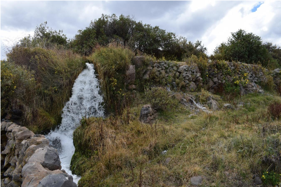
Figure 3.12 Irrigation water exiting a canal at a water drop and leaking from stone-lined canal edge onto sloped tread, July 23, 2019 (photo by Author).
