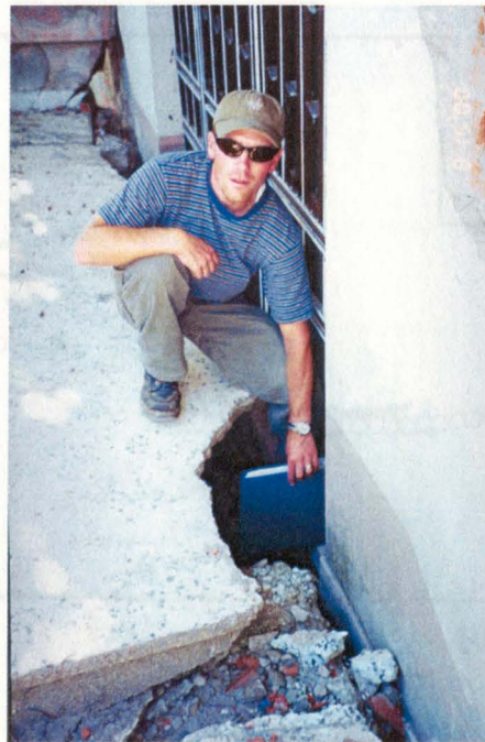
Figure 3.41 Photograph showing approximately 30 cm of settlement between the stairs and the doorway of building N-1 at Site 1-11.
