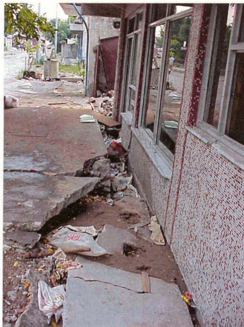
Figure 3.26 Photograph of building D1, which settled and translated during the earthquake. Notice the liquefaction ejecta next to the building (from www.eerc.berkeley.edu/turkey/adapazari ).
