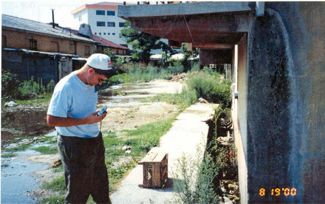
Figure 3.17 Photograph of building C2, which translated 57 cm towards the street (right). Notice the gap between the building and the sidewalk.
