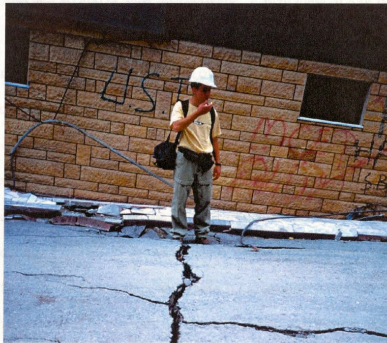
Figure 3.7 Photograph of building A1 showing the severe tilting that occurred when its northwest corner settled approximately 1.5 meters (from www.eerc.berkeley.edu/turkey/adapazari ).
