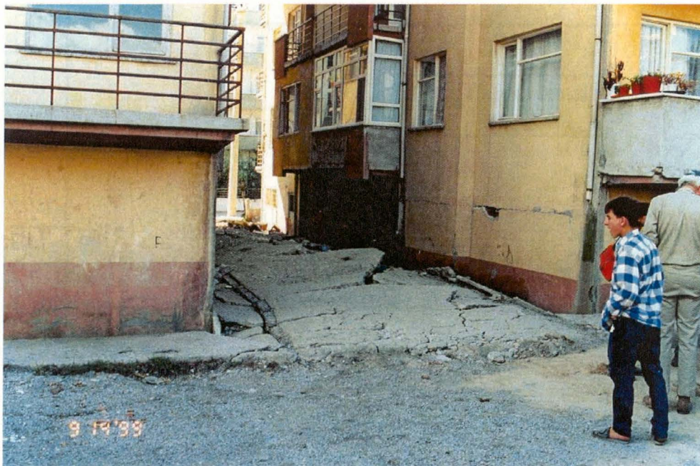
Figure 3.18 Photograph of the alley between buildings C1 and C2, which was crumpled by settlement and translation of the buildings (from www.eerc.berkeley.edu/turkey/adapazari ).
