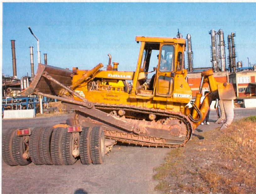
Figure 3.3 Photograph of the bulldozer used as a source at liquefaction sites where deep profiling was desired.
