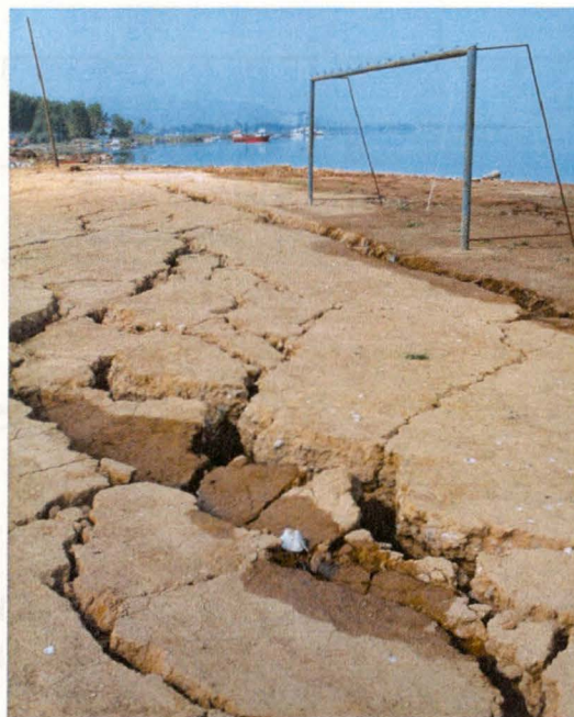
Figure 3.83 Photograph showing the ground cracks caused by lateral spreading into Izmit Bay at Soccer Field (from www.erc.berkeley.edu/turkey/adapazari ).
