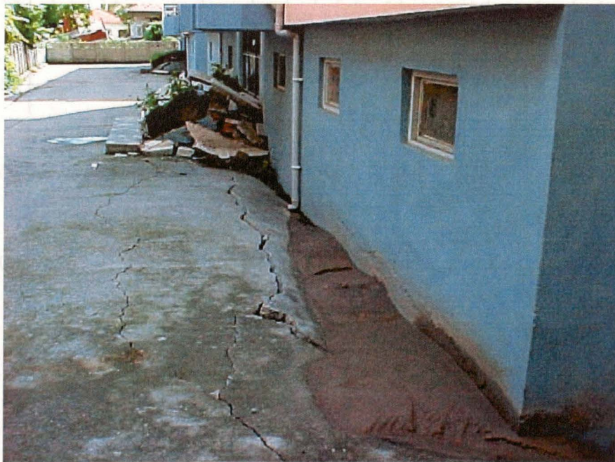
Figure 3.36 Photograph showing the liquefaction-induced settlement at Site J. Notice the liquefaction ejecta (from www.eerc.berkeley.edu/turkey/adapazari ).
