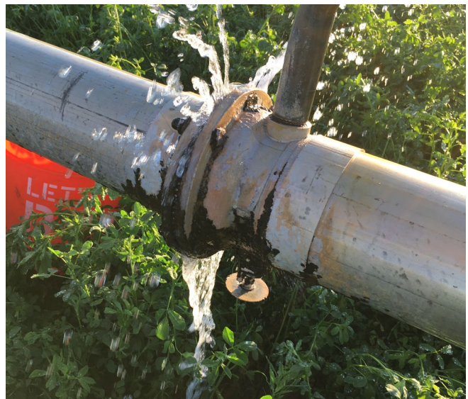
Figure 10. Leaking Joint on a Wheel Line System
