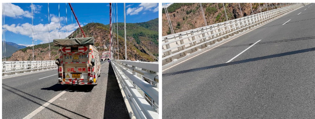
FIGURE 9 Rutting depth detection on the bridge deck pavement.
