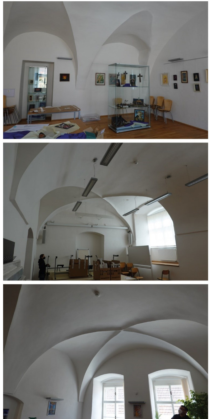
Fig. 1. Barrel vaults with lunettes under room 1.11 (top), cross vaults under room 1.11 and room 1.12 (middle), barrel and cross vaults under rooms 1.17 and 1.18 (bottom). (Photo: Válek, 2021)
