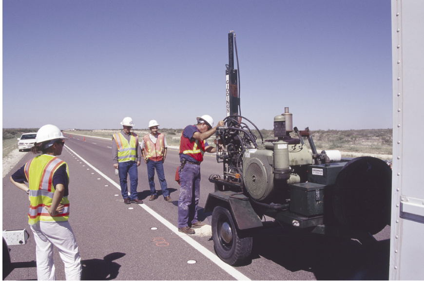
Figure 5. Bureau staff augering through pavement at SRBA site on I-10 in Pecos County, Texas.
