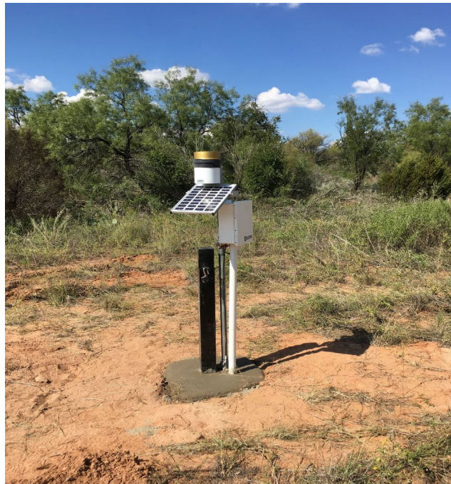
Figure 2. Representative monitoring site, including solar panel, rain gage, and data-logger. Site shown is enclosure at DMF1 middle terrace well.
